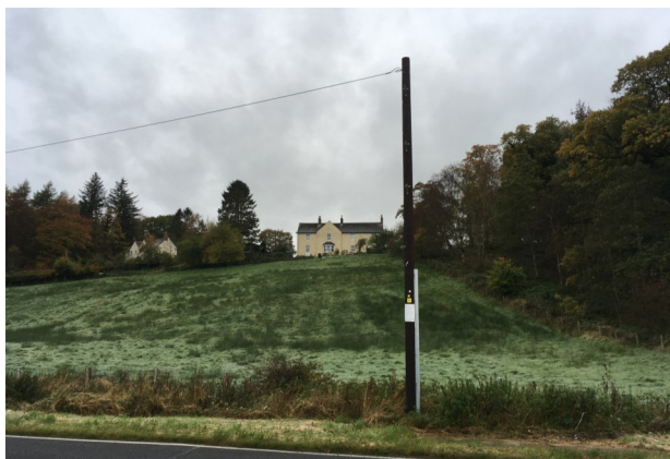
Fibre connection via telegraph poles
