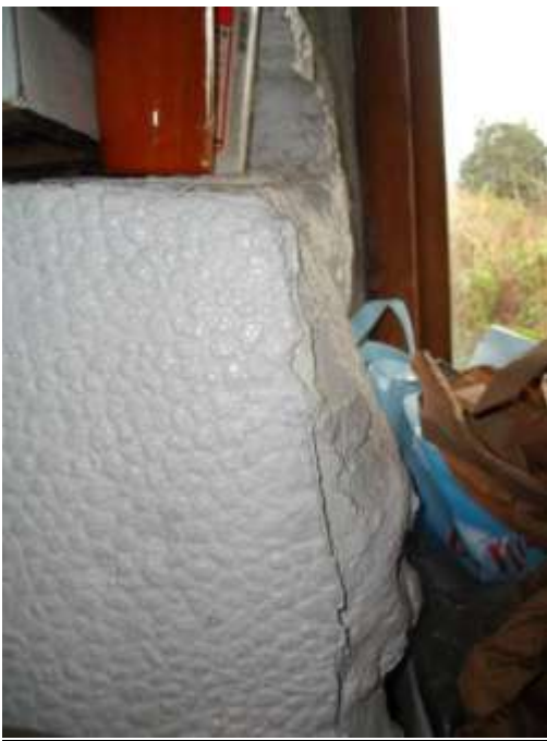
Above: An example of bespoke insulation
