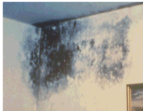
Condensation & black mould in the corner of a room
